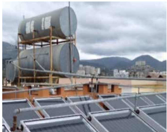
FIG. 2. Hot water storage tanks supplied by a central solar heating system in the block of Patient 1
